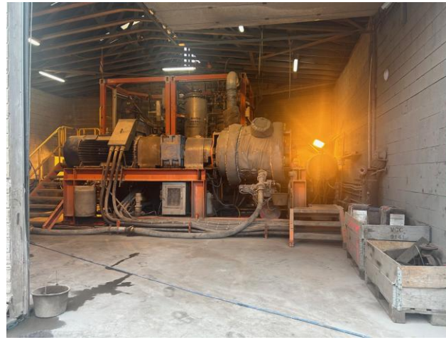
Heating Process to Separate Base Oil / Drilled Cuttings
